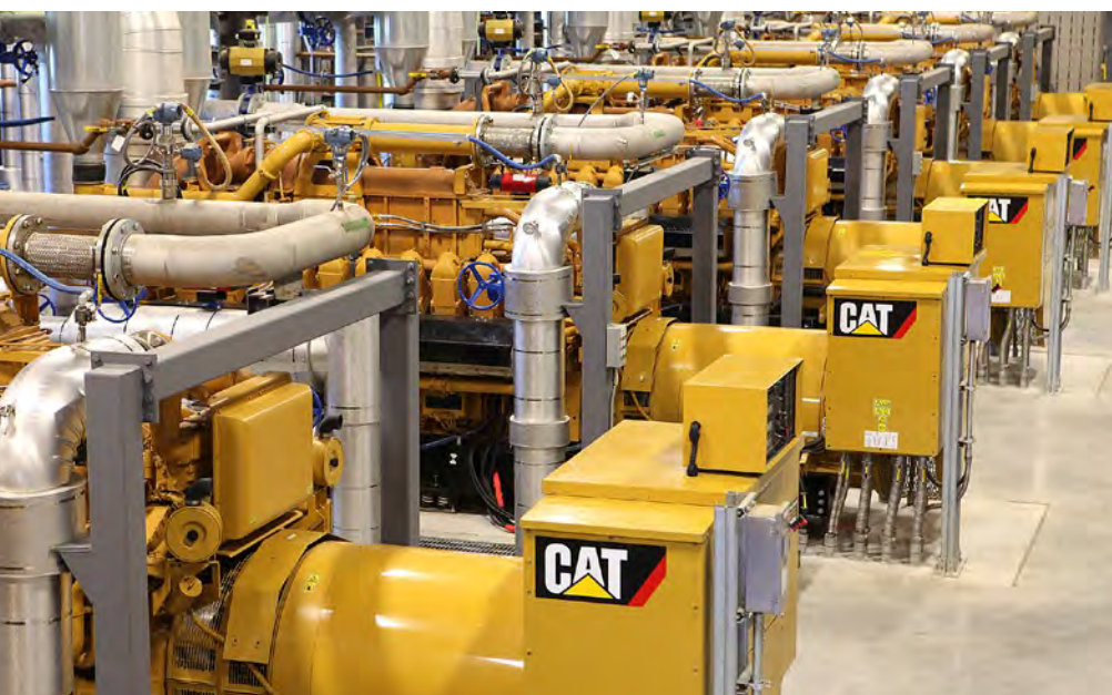
Cat® generator sets installed at a landfill gas processing and power plant near Montreal, Canada, producing electricity from landfill gas.
