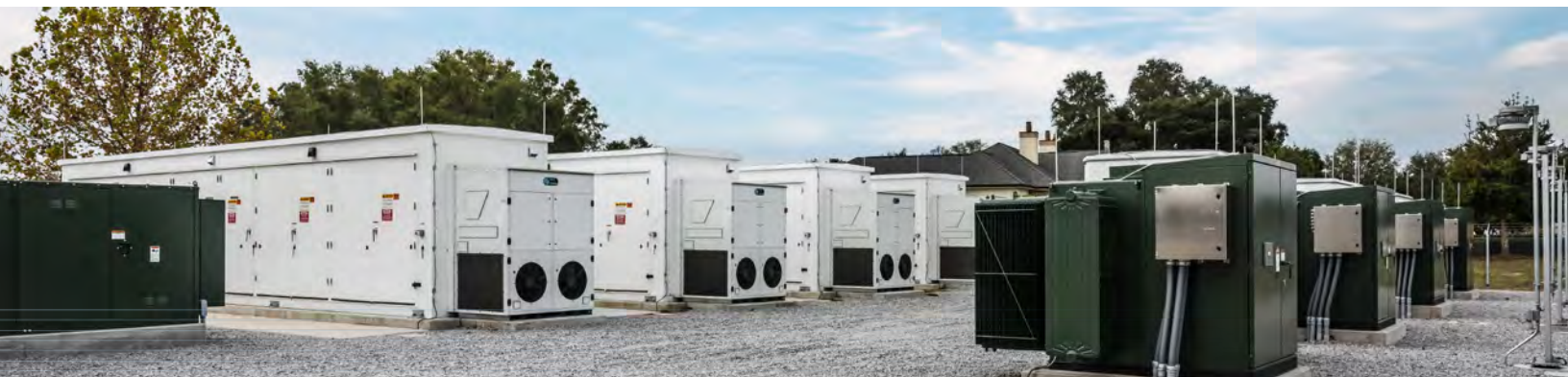
Trenton Battery Storage Facility / Trenton, Florida
