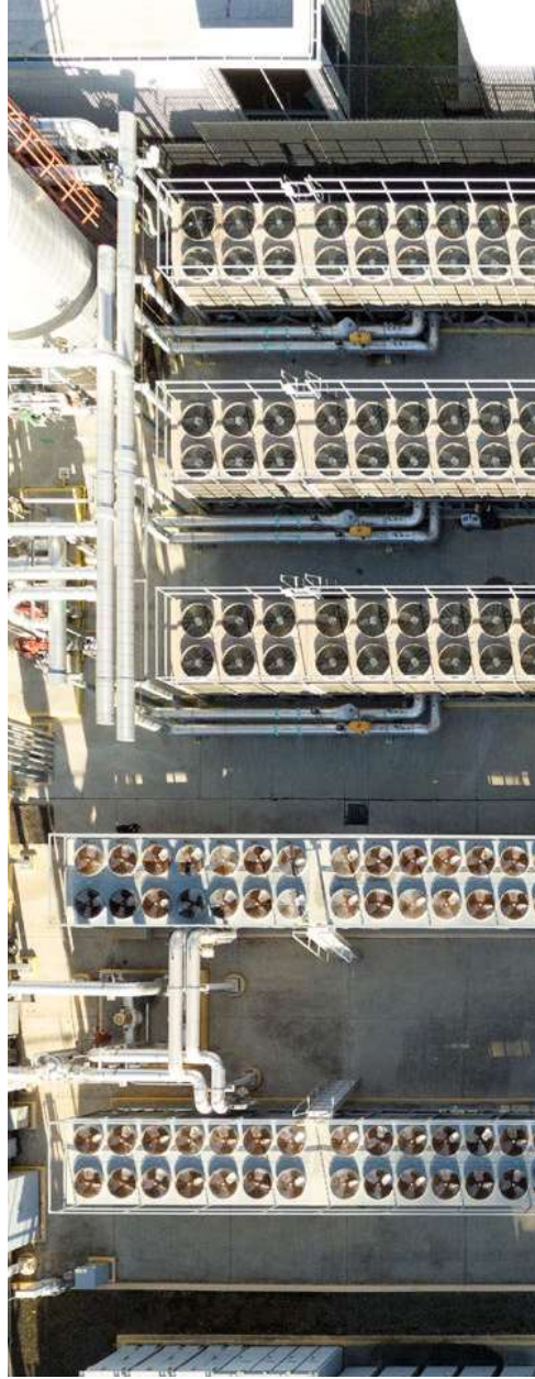
Cooling system at Intel's Mission Campus in Santa Clara, California.
