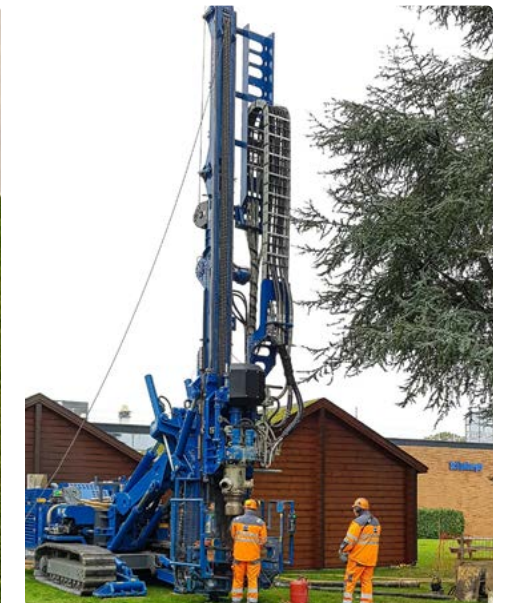
Celsius Energy installation (above) and final surface footprint (left) at the Schlumberger Riboud Product Center in France.
