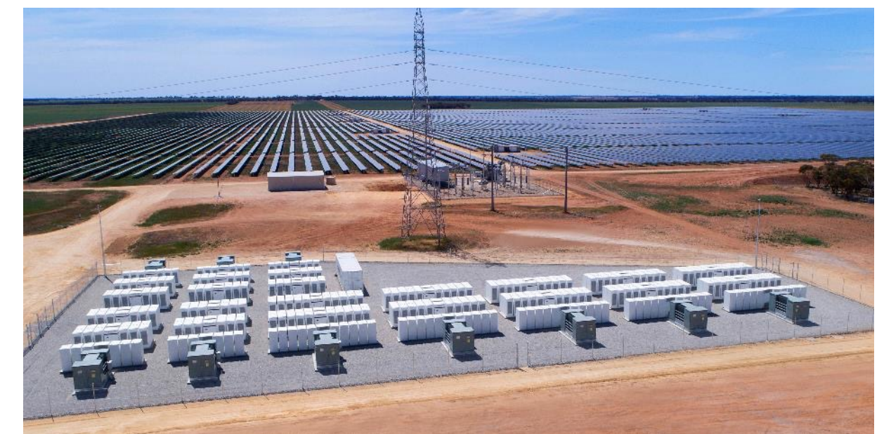
Commercial Solution: Solar and Storage
